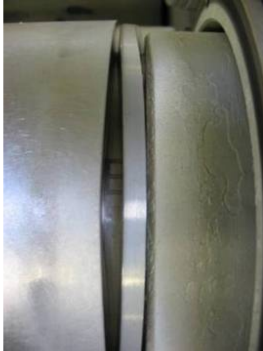
Figure 5. Deformed Welded Retaining Ring with Sleeves Mounted
